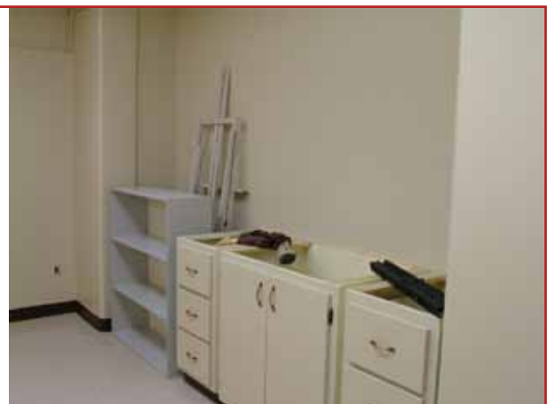
CABINETS TO BE INSTALLED IN THE NEW ROOM.
